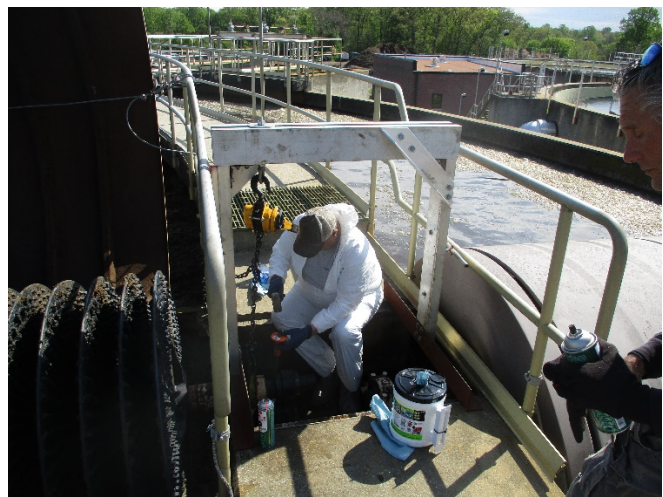
Repairs to Aerators & Replacement of over 700 Aeration Disks Orbal Oxidation Ditch Cell #2 Repairs
