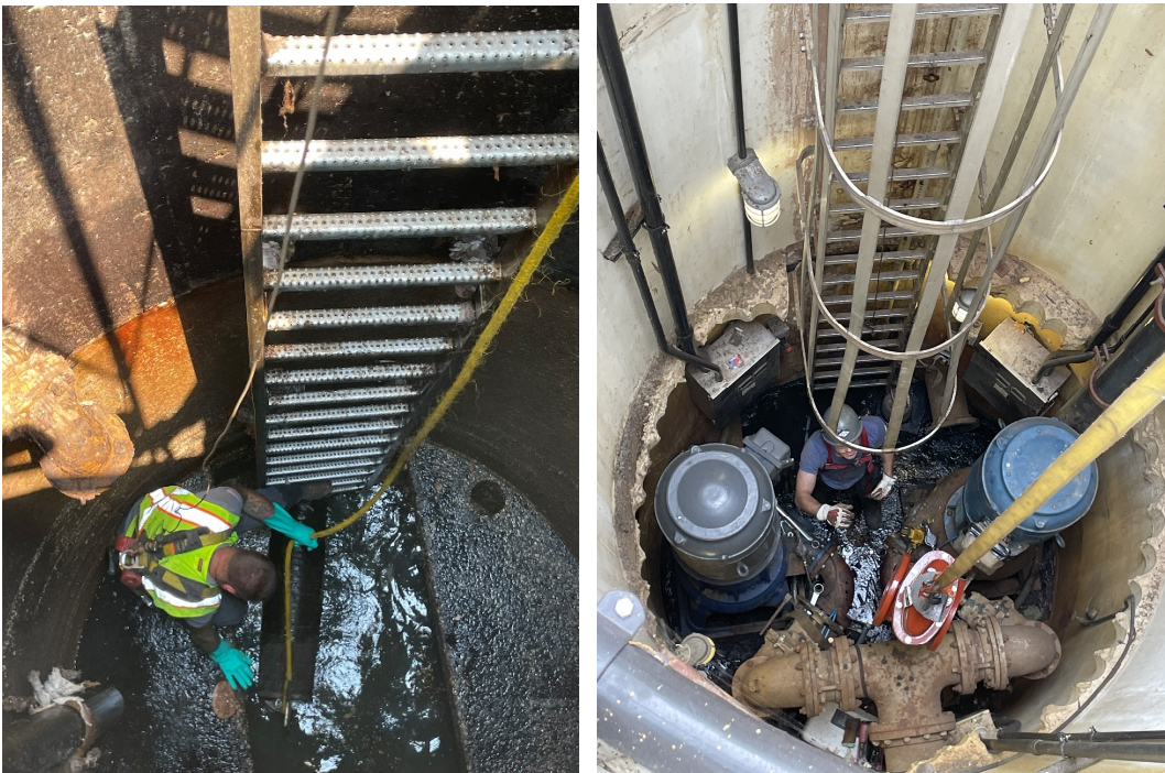
Valve rehabilitation and replacement work in the wet well and dry well of the Authority’s Birchfield Pump Station (1 of 41 Pump Stations)
